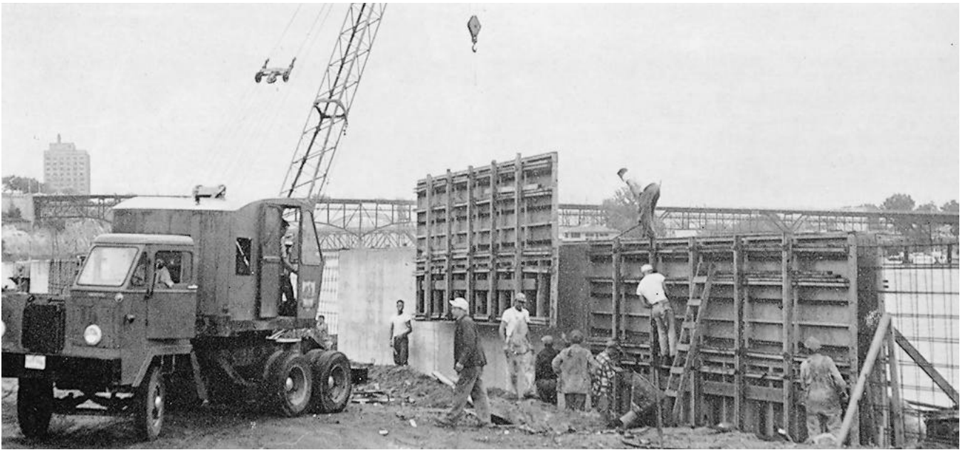
In gang forming, shown here, whole units are lifted into place at once—a technique which saves costly manhours.
