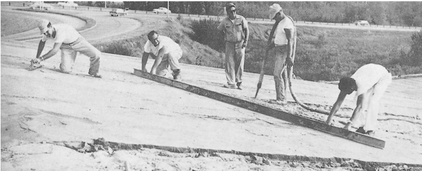
Pumping a 1:6 mix of vermiculite insulating concrete 4 inches thick on the gable roof of a supermarket. Almost any architectural requirement can be met by changing the type of form, slab thickness, concrete mix or support spacing, and steep inclines can be dealt with readily.
