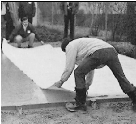
Vacuum mats protect the slab during a sudden rain and permit dewatering to be done during a storm; finishing operations require a period virtually free of precipitation.
