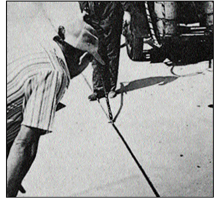
To seal properly, the operator holds the sealing tip at the bottom of the joint and fills the joint with sealant to a level \frac{1}{4} inch below the pavement surface.
