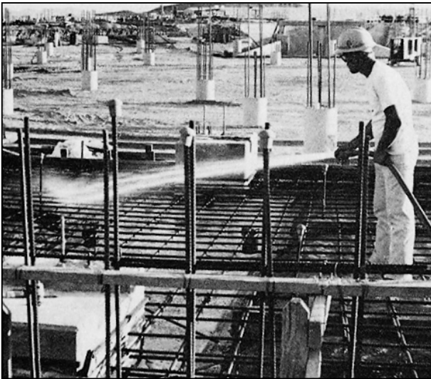
Worker carefully sprinkles formwork and reinforcement to lower temperatures just ahead of the concrete placement.
