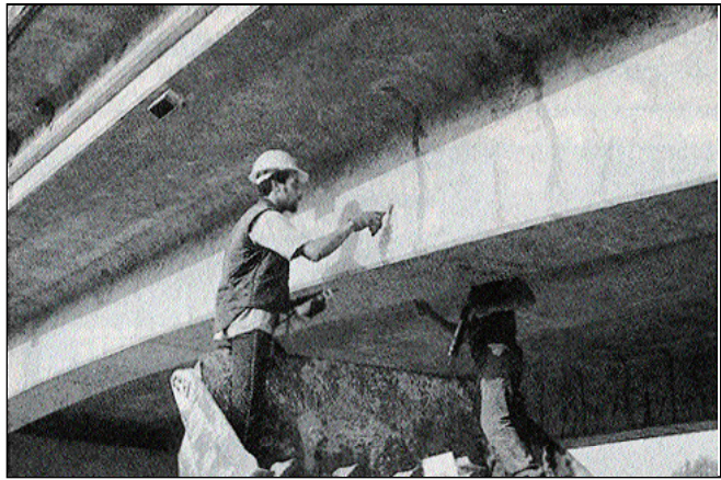
Cracks on surface of girders are sealed with silicone before drill holes are injected with epoxy.
