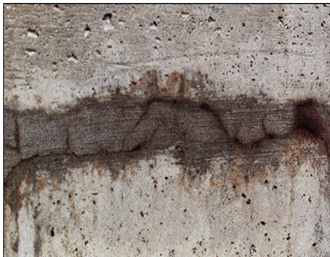
Figure 1. Materials that shrink excessively won't bond well to existing concrete. Shrinkage cracking and loss of bond caused this mortar patch in a wide crack to fail.
