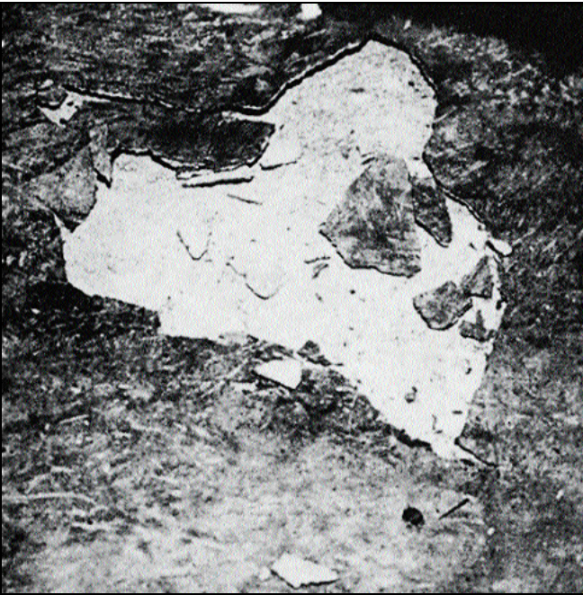
Figure 4. An impermeable but otherwise good quality epoxy overlay lost bond because moisture rising through the slab on grade built up pressure under the impermeable overlay.
