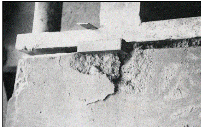
Figure 3. Lower modulus grout beneath the machinery base plate deformed excessively, placing all of the load onto the stiff steel shims that were improperly left in place. As a result, the underlying concrete failed.
