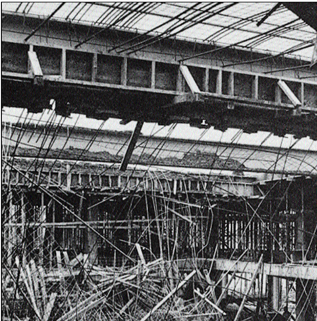
Figure 2. Formwork for concrete cast around steel girder remains in place, suspended from the girder (see cross section in Figure 1) while double-deck shoring has toppled to the ground. Metal post shores were used on this job, but similar difficulties with double-decked wood shores have been experienced when proper bracing has been neglected.
