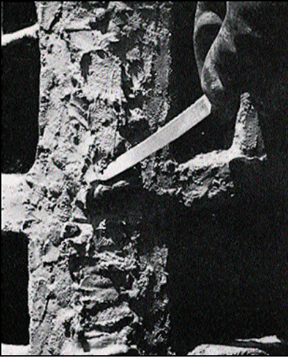
7 The joint between the sections was filled with white-cement mortar, and the fresh mix was given a rough texture with a bent knife blade. Similar mortar texturing was done on foundation surfaces to match the sculpture.
