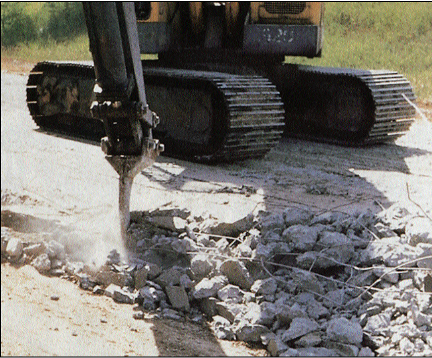
Figure 3. Attached to a backhoe, a rhino horn rips reinforcing steel from the pavement and windrows broken pavement on the grade.
