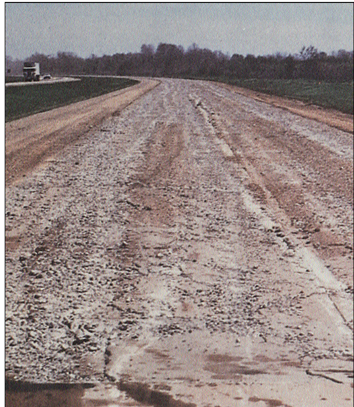
Figure 2. Workers used a 30,000 foot-pound pile hammer pavement breaker to break this pavement. Particles look rather fine in places, but in general pieces are about 2 to 3 feet in size.
