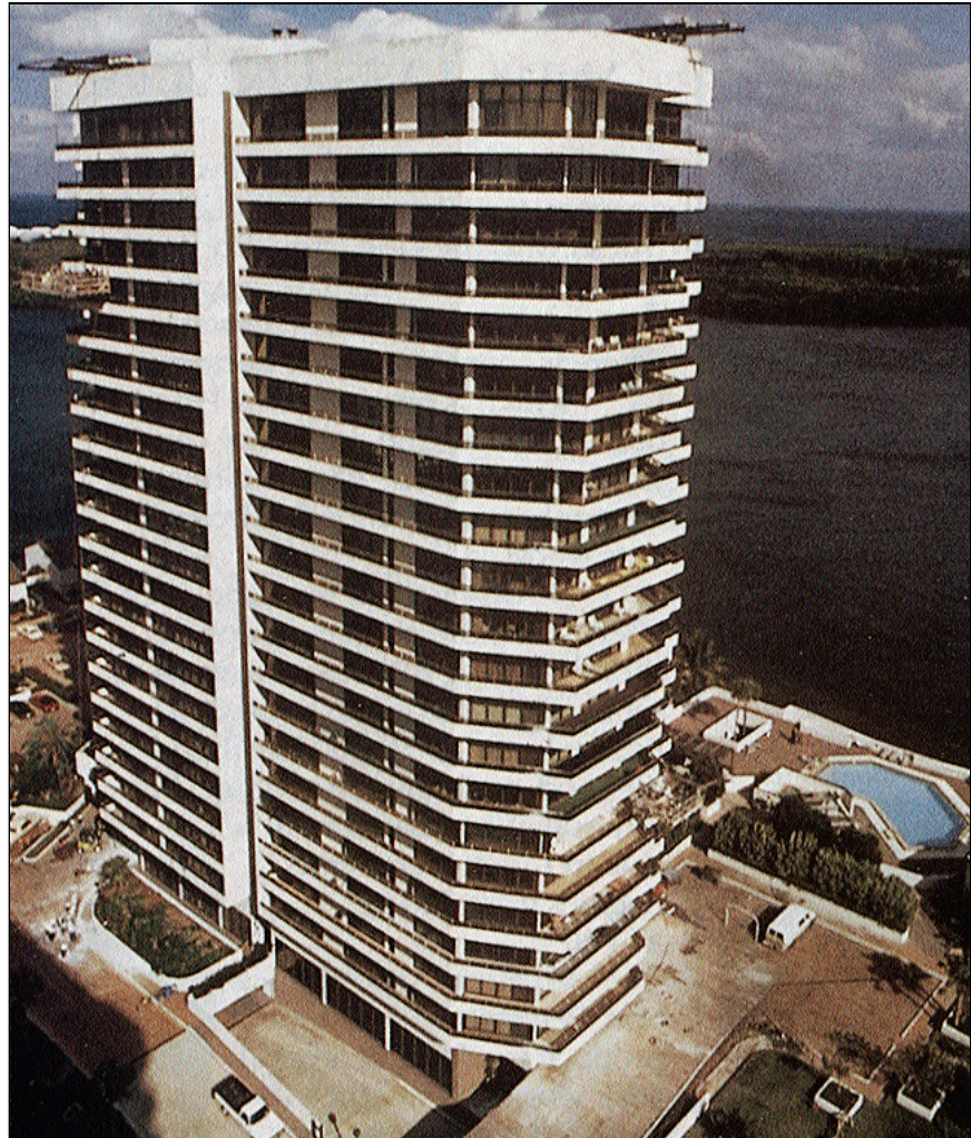
Figure 1. The 8½ -inch-thick concrete balconies that run around the perimeter of this residential building in Florida had cracked and sagged. The scaffolding for the repair is hung from the roof.
