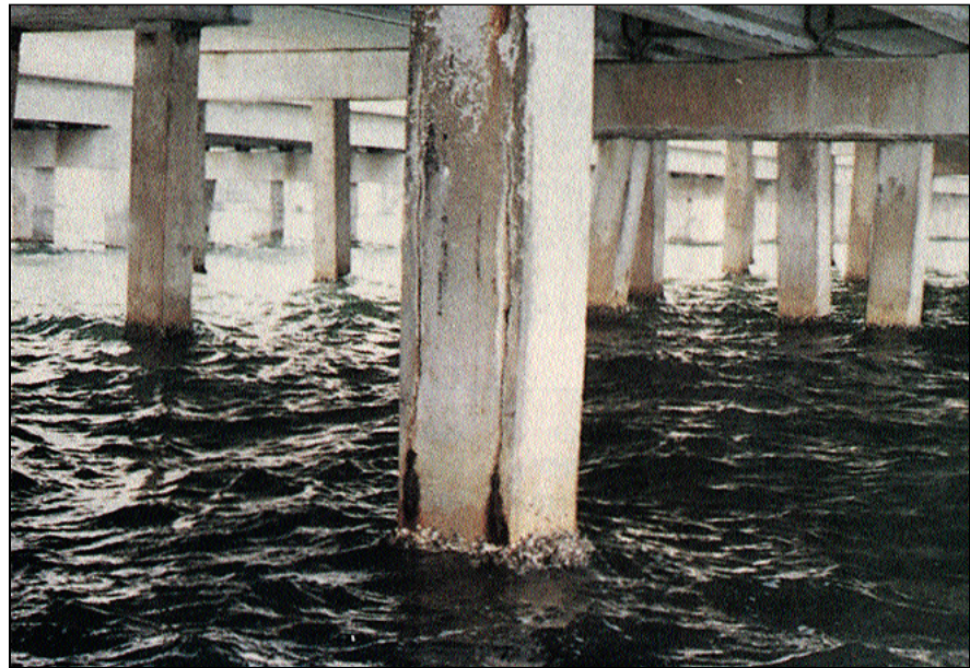
Seawater causes both chemical and physical deterioration processes to concrete. Choosing a high-strength, low-permeability concrete mix increases the service life of the concrete in a marine environment.
