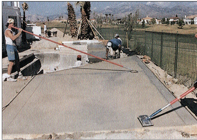
Figure 2. Workers use special edger/jointer tools to cut bordering strips in fresh concrete. These strips will be patterned differently from the inside areas.
