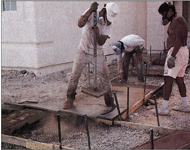
Figure 3. The bands of concrete in this walkway are being patterned before the larger concrete sections are placed. On detailed projects, separate pours can make it easier to place concrete of contrasting patterns or colors. Workers wear particle masks so they won't inhale powdered release agent.
