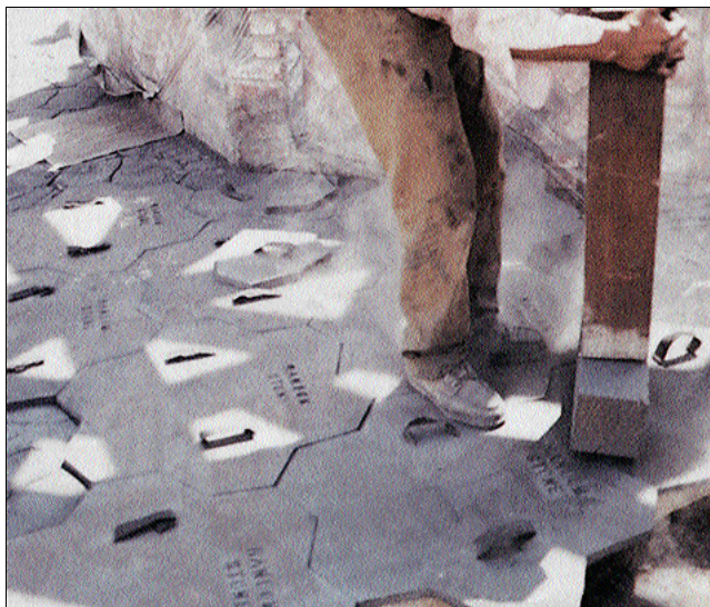
Figure 1. After placing the stamping tools, tamp them using just enough force to impress the texture into the concrete surface. Notice that the brick walls in the background are covered with plastic to prevent accidental staining from the coloring agents.
