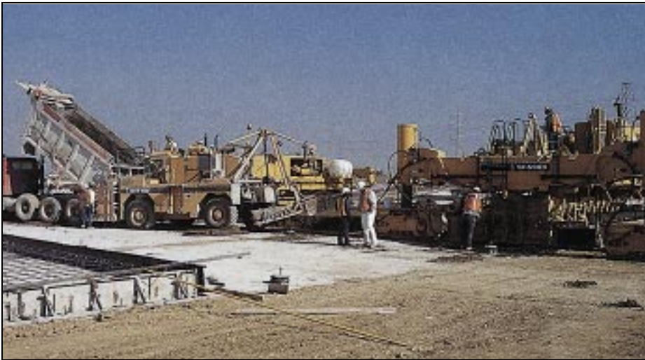
A rubber-tired material transfer/placer with a pivoting, rear-mounted conveyor places concrete in the first few feet of a paving lane.
