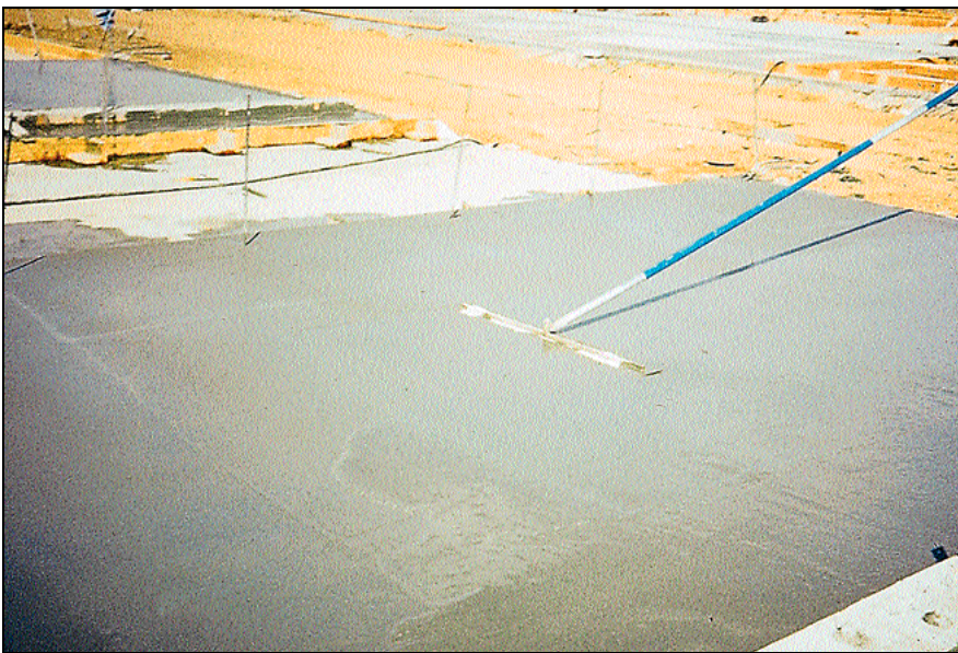
Using a fresno while the concrete is still bleeding seals the surface. This stops further bleeding but traps bleedwater beneath the surface and can cause blistering, surface delamination, or deicer scaling. Wood floats, which work best on non-air-entrained concrete, keep surfaces open, so bleedwater isn't trapped beneath the surface.
