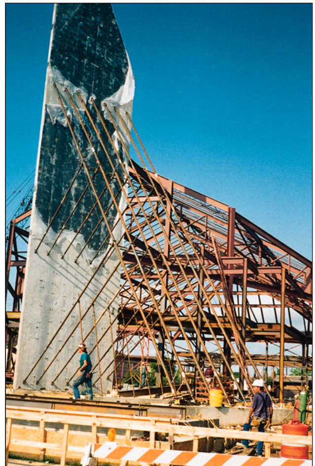
Figure 3. Extensive bracing was needed to support each panel. The seven 62-foot-long main braces had knee bracing at two locations. And even the longest knee brace required bracing.
