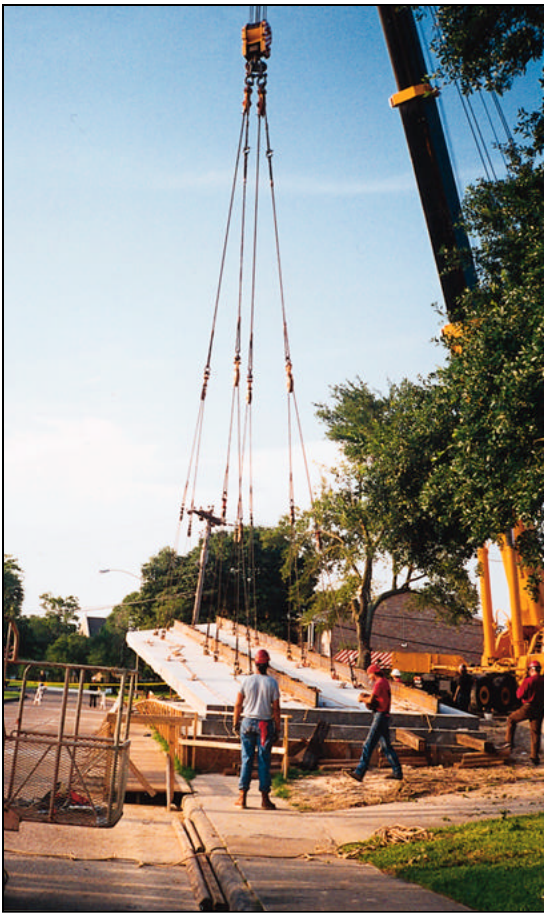
Figure 2. Each panel had 8 high by 2 wide (16-point) rigging to accommodate bending stresses produced by lifting.
