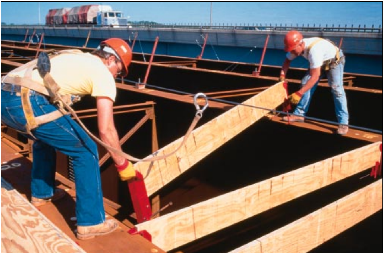
Workers set LVL beams into adjustable joist hangers to support deck forms from the girders of a steel bridge.
