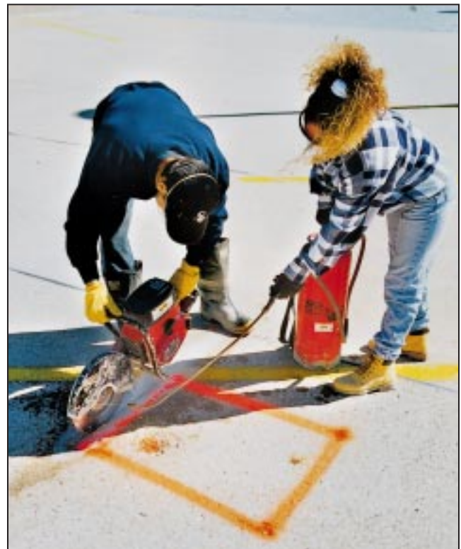
Figure 3. Sawcutting the perimeter of the patch establishes concrete removal boundaries and prevents feathering.
