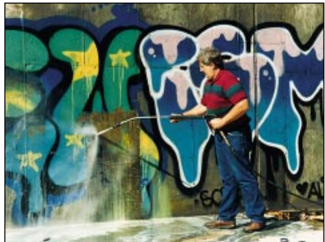
Power washing can be used with various chemical strippers to remove graffiti.
