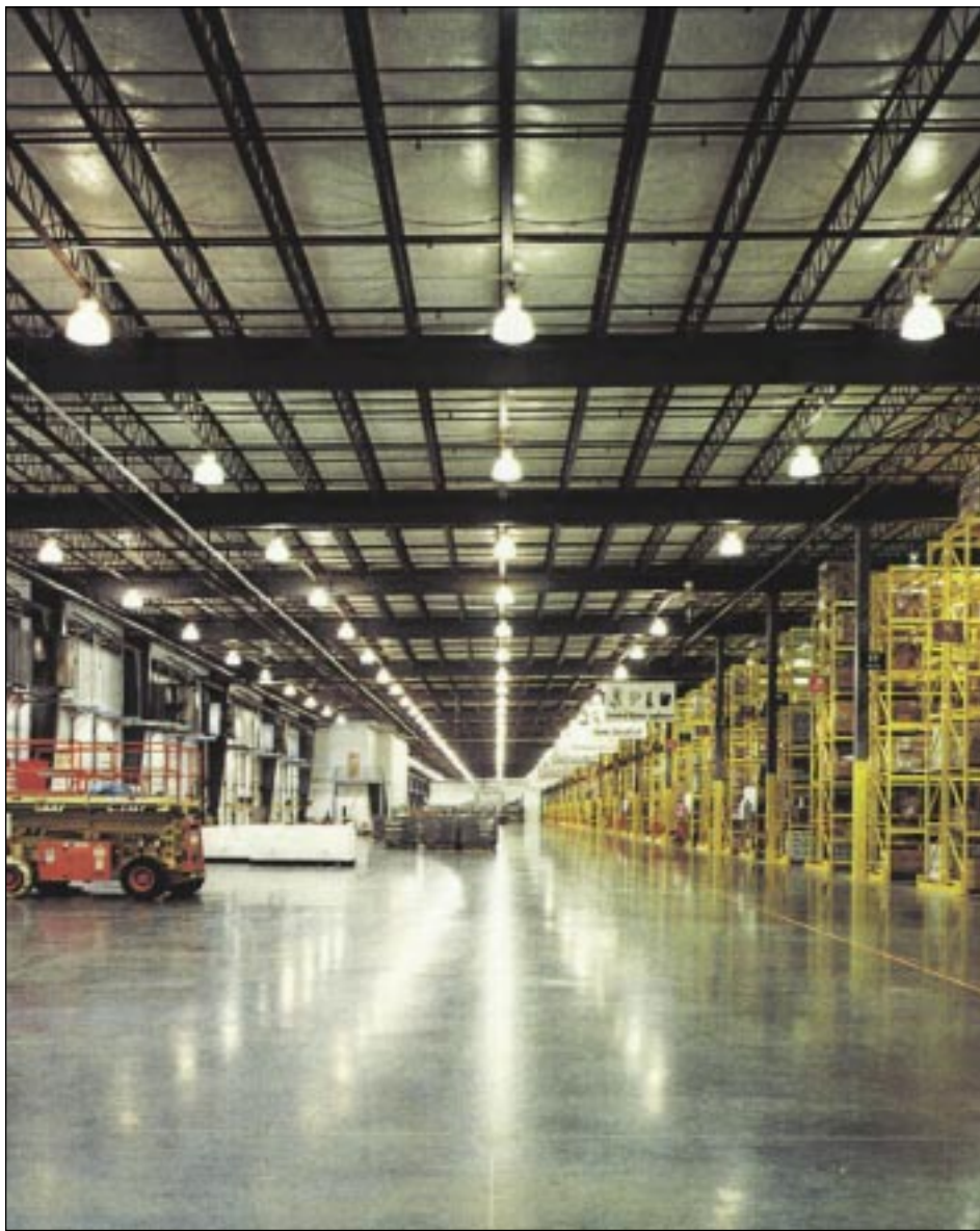
A year later, the floor is free of cracking and curling.
