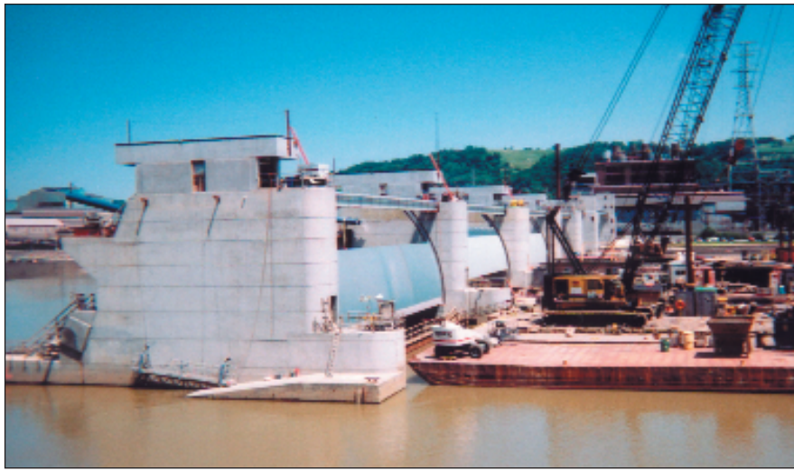
Gate installation on the new Braddock Dam, where precast segments that were floated in, set down, and filled, form the lower third of the pier bases and overflow sections.
