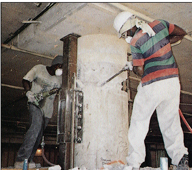
After the roof load is transferred to the lifting posts, a 12-inch-wide segment is chipped out of the column. The reinforcing bars are cut just prior to lifting.
