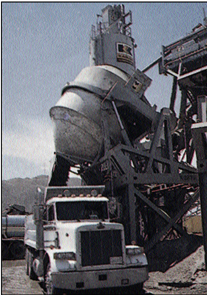
Kasler Corp.'s 12-cubic-yard-capacity mixer discharges a load of concrete into a waiting dump truck. The company has a contract to place 190,000 cubic yards of concrete at Denver International Airport.
