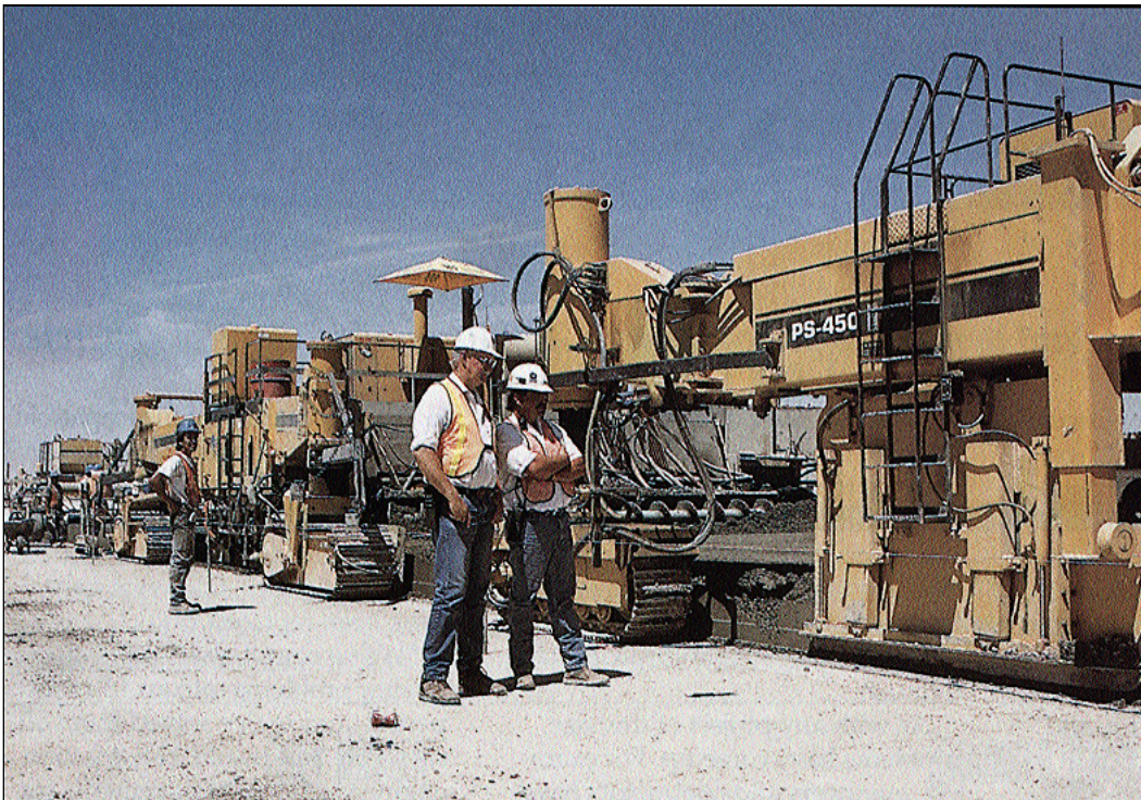
Ken Norin, left, and Randy Hardman observe Interstate Highway Construction's paving train: a placer-spreader, paver, and texture-cure machine.
