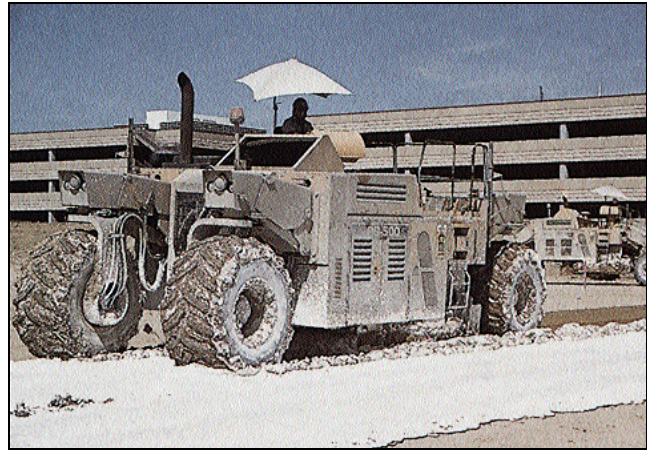
A reclaimer-stabilizer incorporates lime into subgrade for Mt. Carmel Sand and Gravel at a Denver International Airport parking lot.
