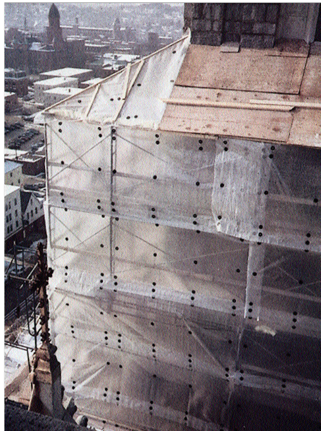
Clear plastic sheeting allows the sun to light the enclosed work area. Grommets are used to join sheets or attach the sheeting to scaffolding or 2x4 framing.
