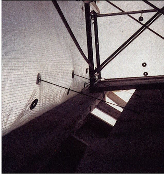
Flexible ties and cords attach the sheeting to scaffolding rails, planks, or timber framing for the enclosure.
