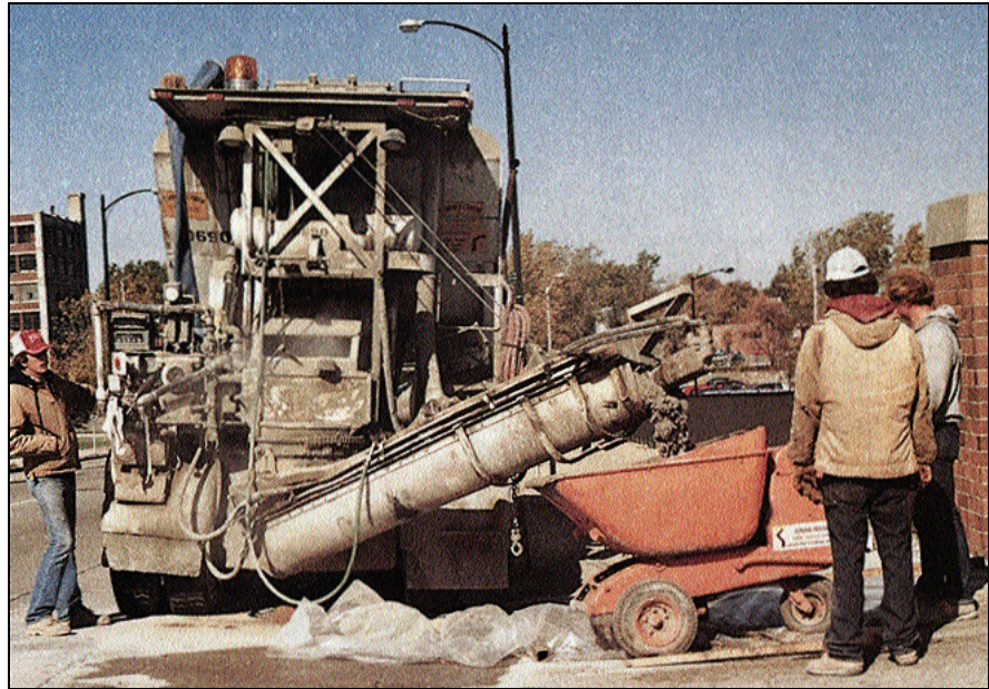
Figure 1. You must make LMC onsite. Most contractors use a mobile batcher mixer; it holds all the raw materials for LMC on board and it can run continuously or as needed.
