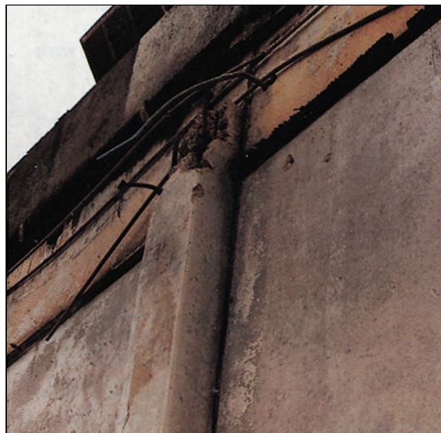
View of the top of a concrete pilaster shows where a girder pulled away from the pilaster before collapsing.
