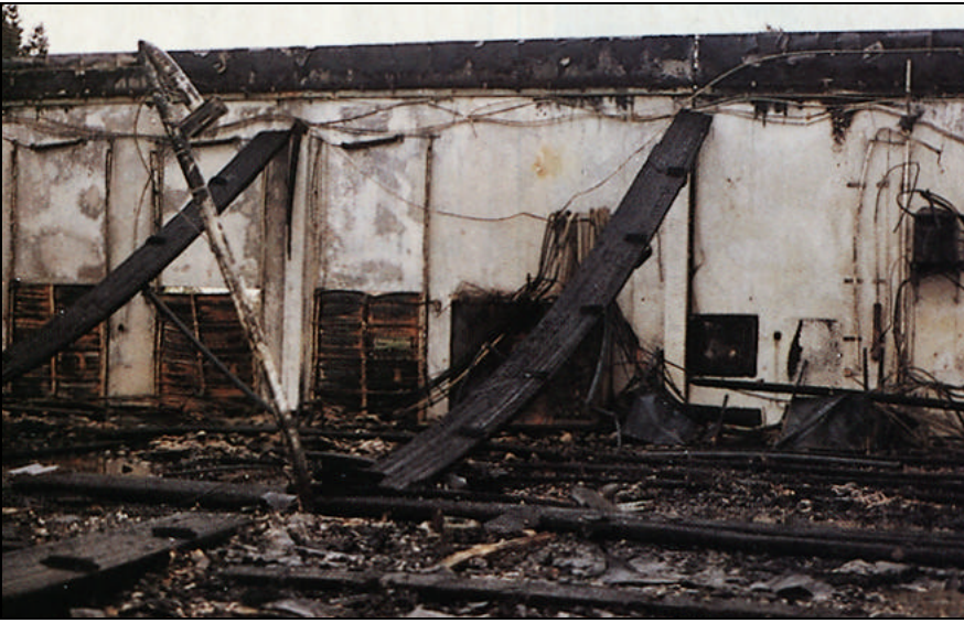
Interior view of the building shows the extreme damage caused by the fire. Little remained of the plywood roof system except for the glue-laminated girders. Here two collapsed girders are leaning on the tilt-up wall panels. The steel pipe columns supporting the girders buckled in the intense heat. One such column appears in the left side of the picture.
