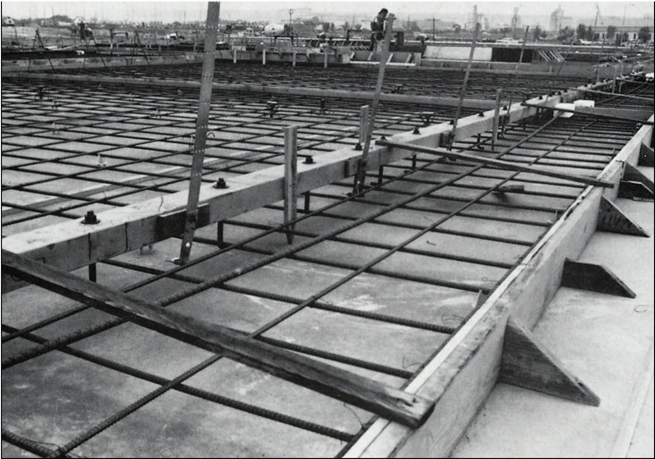
Seismic straps protrude from this panel, which is ready for placing concrete.
